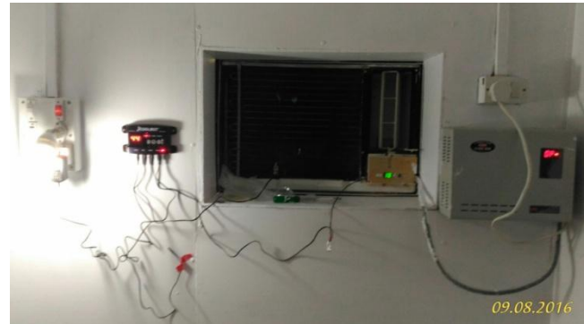
Fig. 3 Working of CoolBot system
